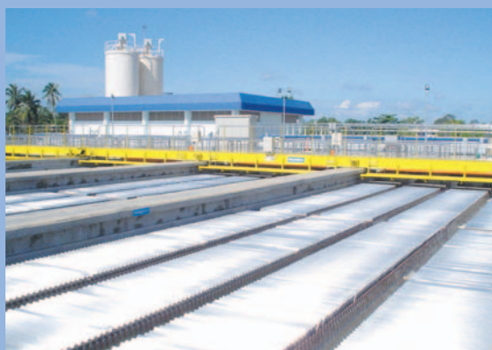
Lamella Clarifier installed at Kepong 3 Water Treatment Plant, Kuala Terengganu
