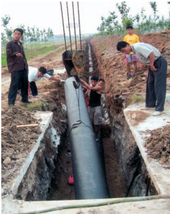
Pipe laying works to new townships for the Changle water supply concession.
