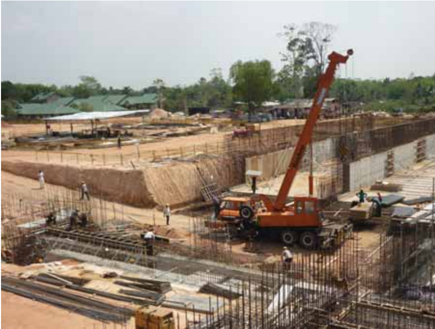
On-going construction works of the 64 mld Kalu Ganga project in Sri Lanka
