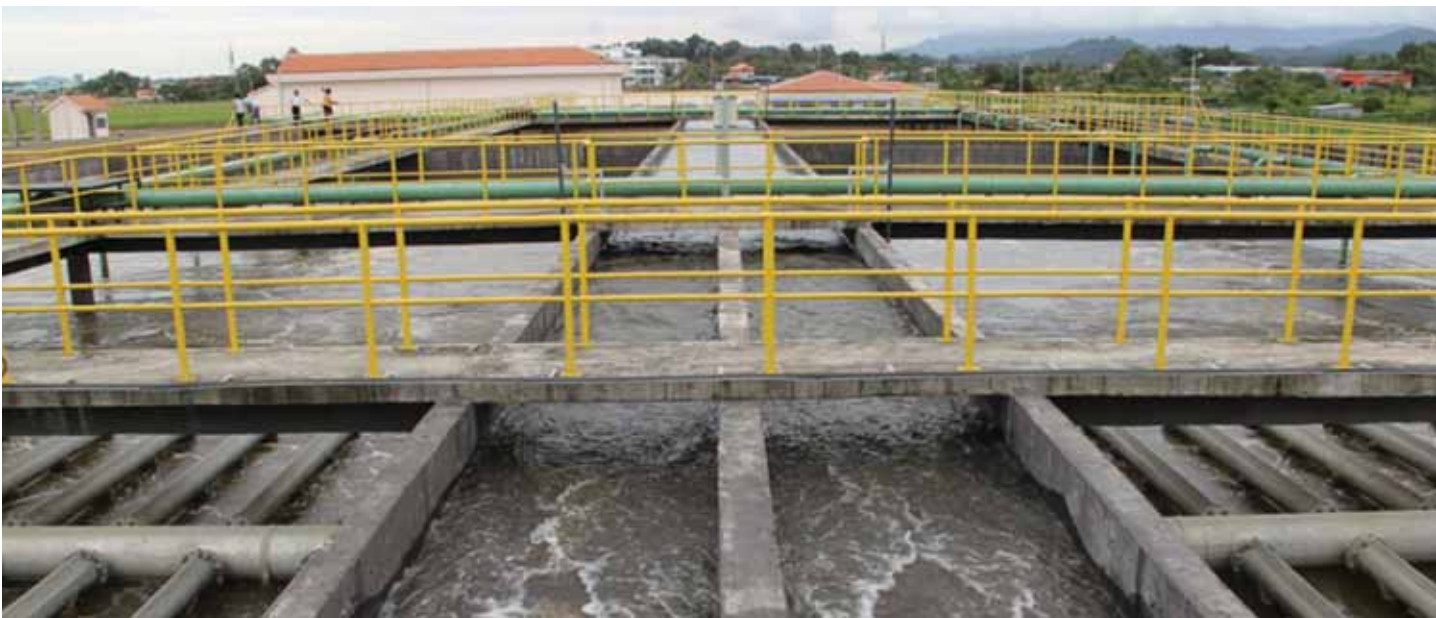
View of Kota Kinabalu Sewage Treatment Plant with Phase 1 capacity of 75,000 population equivalent.
