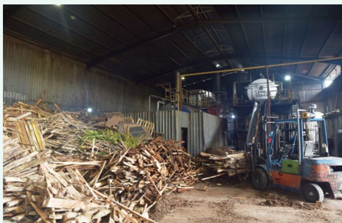
Generation of steam energy by using wood biomass through combustion at JREMT
