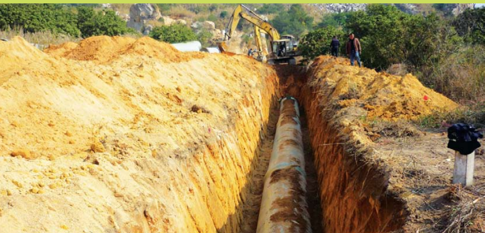
Pipe laying work in progress for the 175 mld Nan An Raw Water Supply Project, Nan An City, Fujian Province, China
