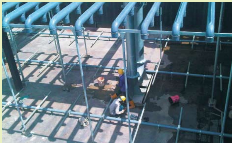
Installation of decanters and aeration pipes for Penampang Regional Sewage Treatment Plant with ultimate capacity of 300,000 PE for the Kota Kinabalu Sewerage Project Phase 1, Sabah
