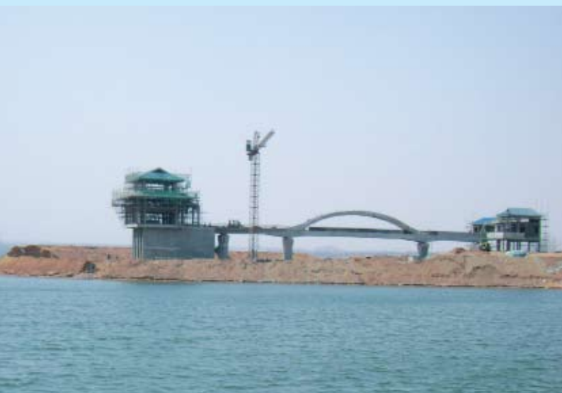
Intake structure works in progress at the new 100 mld Changle Raw Water Project, Changle County, Shandong Province, China
