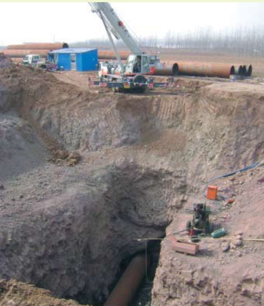
Laying of pipelines in progress at the Changle Raw Water Project, Changle County, Shandong Province, China
