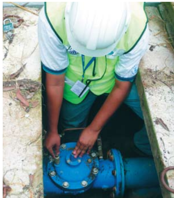
Maintenance and Servicing of Pressure Reduced Valve (PRV)
