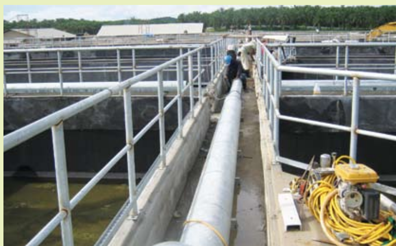
Installation of air pipe for aeration tank in progress at the construction and completion of infrastructure works for Medini Development, Iskandar Malaysia, Johor
