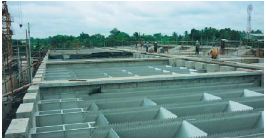
Filtration plant construction in progress at Kelani Right Bank Water Treatment Plant, Sri Lanka
