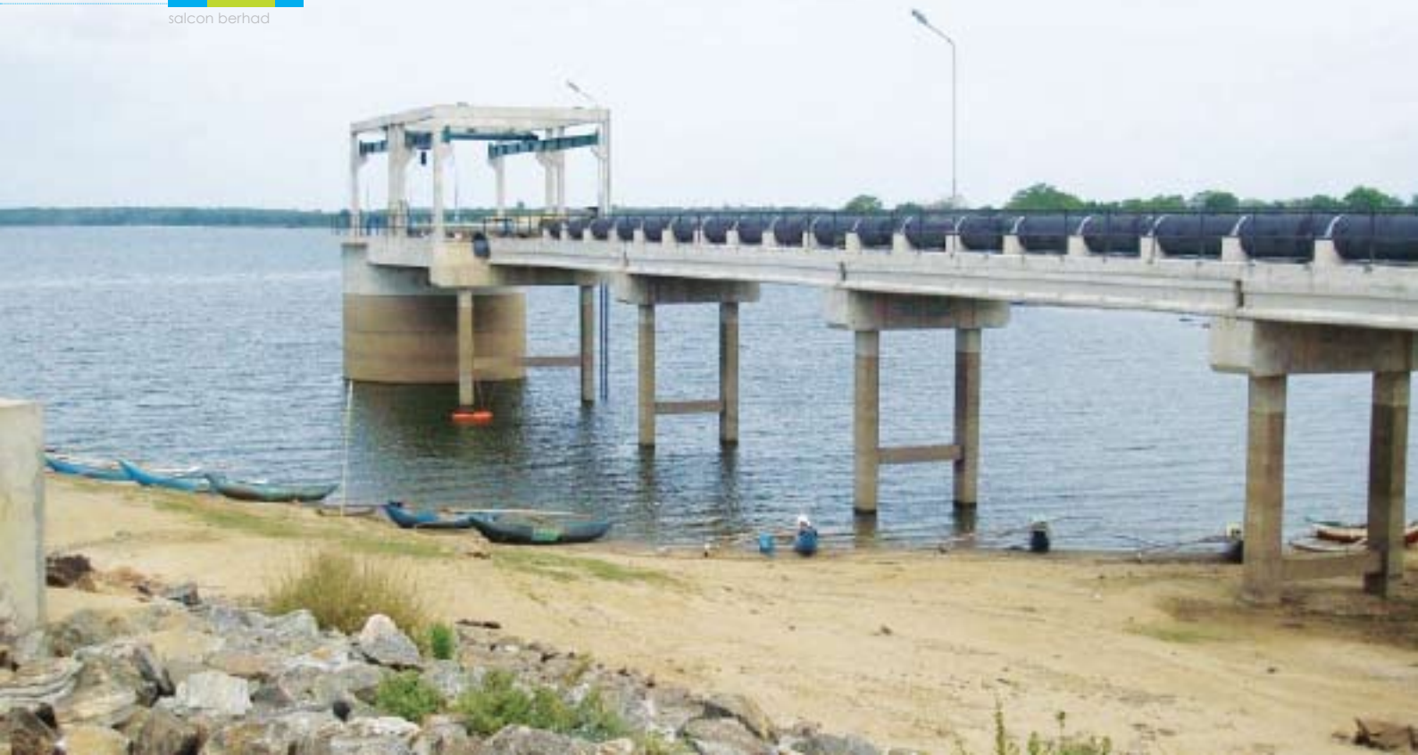
View of Raw Water Intake at the Batticaloa Water Supply Project, Sri Lanka
