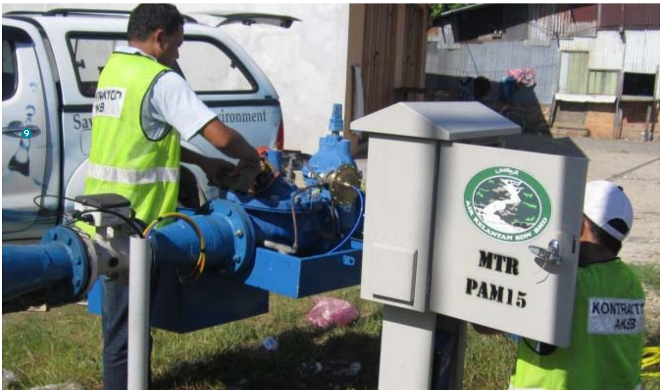
9. Maintenance Service at DMA Meranti B, Pasir Mas, Kelantan for Kelantan NRW Project.
