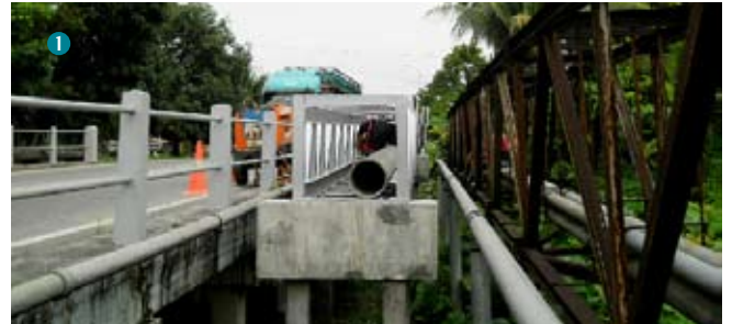
1. Main Pipe Installation at Bukit Jawa, Pasir Puteh, Kelantan for Kelantan NRW Project
