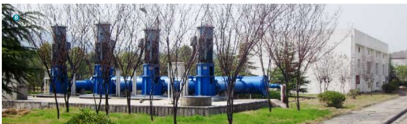
8. Charging pump at Wukang Water Treatment Plant with 60 MLD of treatment capacity.
