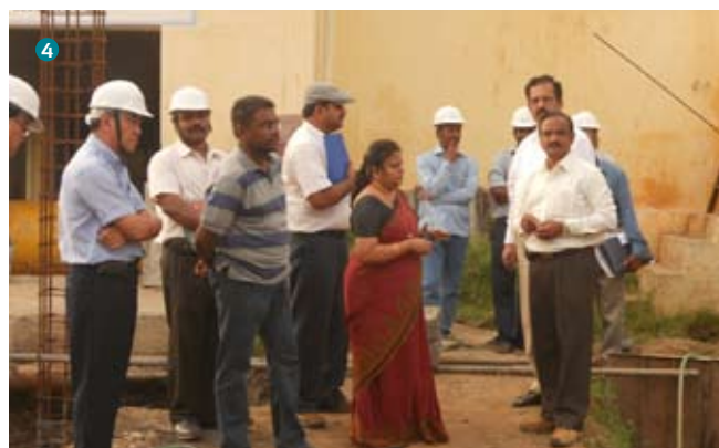
4. Visit by Mayor of Davanagere City to Davanagere's raw pumping station to view the work progress.
