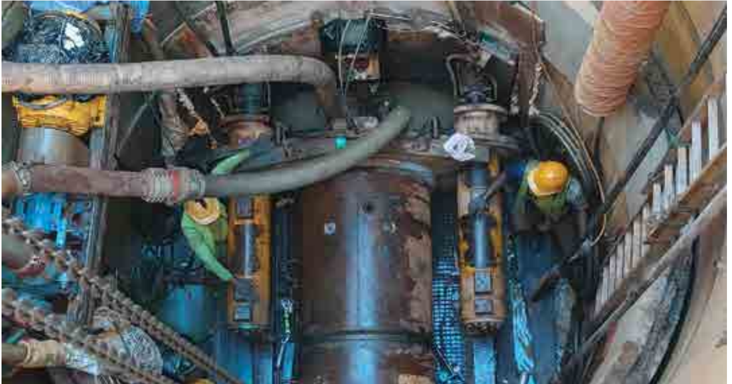
External Common Gravity Sewer Mains, Jalan Segambut
