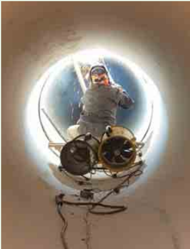
Internal welding of 1400mm ND pipe for Kuala Terengganu Utara water treatment plant.
