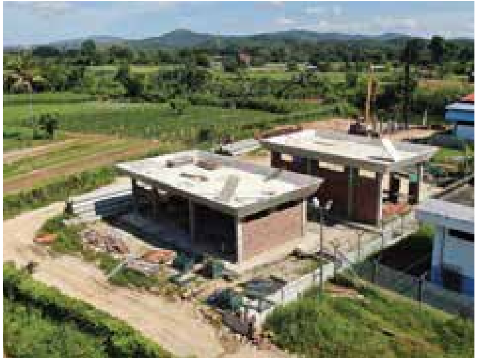
▲ Construction of Consumer Building and Sabah Electricity Sdn Bhd substation in intake boundary at Telibong II water treatment plant
