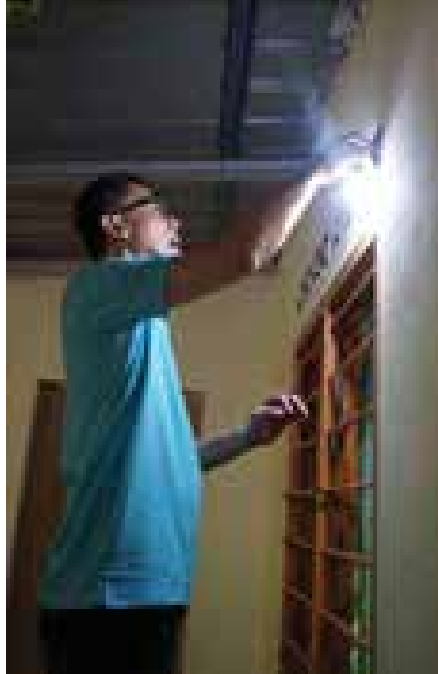
▲ Salcon volunteer installed solar lighting system and light bulbs for one of the identified households
