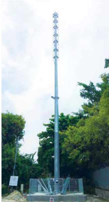
► A 30 meter cell site owned by VBT delivered at Cempaka LRT Station
