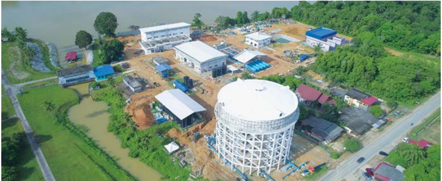
► Overview of Raw Water Intake at Pulau Bahagia, which forms part of Kuala Terengganu Utara Water Supply Scheme
