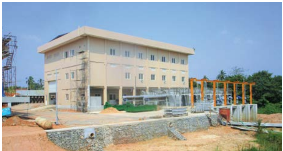
► The design and building of Ambathale Stormwater Pumping Station is expected to be completed in 2021
