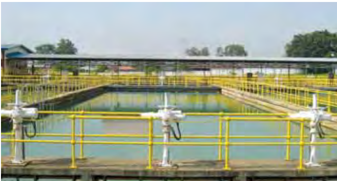
Binh An Water Treatment Plant in Ho Chi Minh City, Vietnam with total capacity of 100 Million Litres Per Day (MLD)
