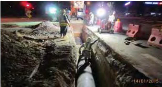
Installation of main pipe at Tropicana Metropark, Off Persiaran Teknologi Subang, Shah Alam
