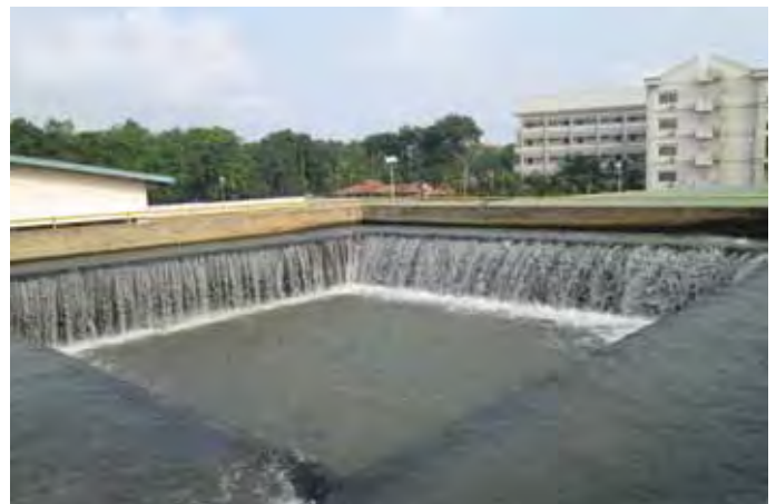
View of Aerator at Binh An Water Treatment Plant, Vietnam
