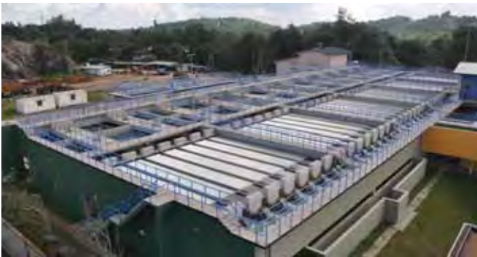
Sedimentation tank at Kelani Right Bank Water Treatment Plant, Sri Lanka
