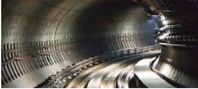
Laying of fibre optic cables along the LRT track in the Klang Valley
