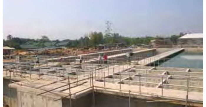
Kandana Water Treatment Plant extension under the Kalu Ganga Water Supply Project in Sri Lanka
