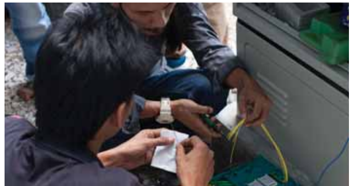
Fibre splicing 1 of 57,000 splices in total during the laying of fibre optic cables along the LRT lines
