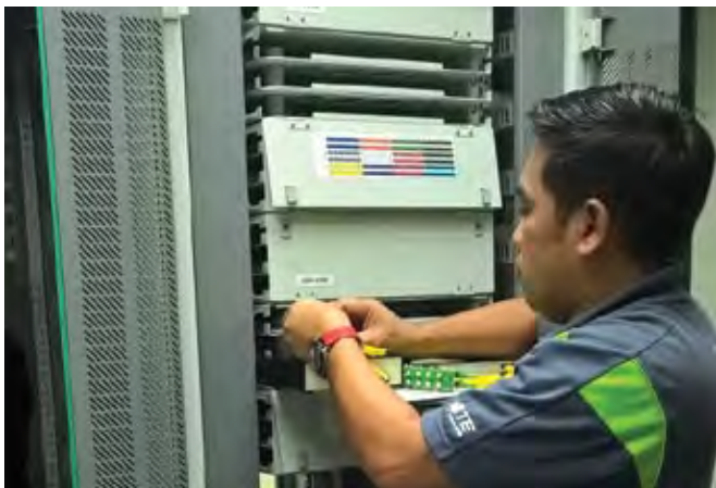
Fibre testing to ensure reliable high-speed connectivity.
