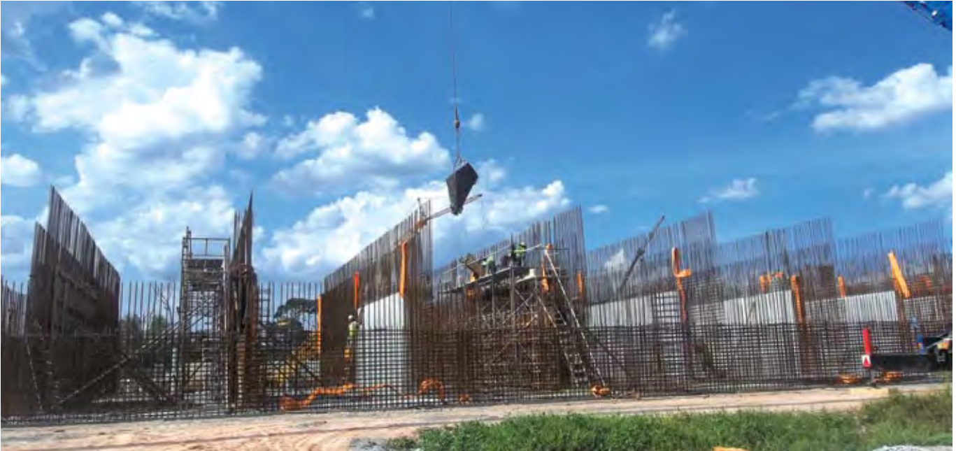
Construction of Secondary Clarifier Wall Tank of Langat Centralized Sewage Treatment Plant.
