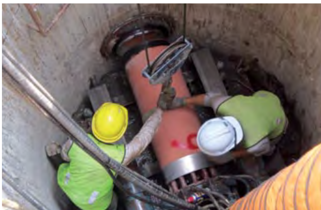
Pipe Jacking earth arrow method is applied to D55 sewerage Pipe Networking project in Klang.
